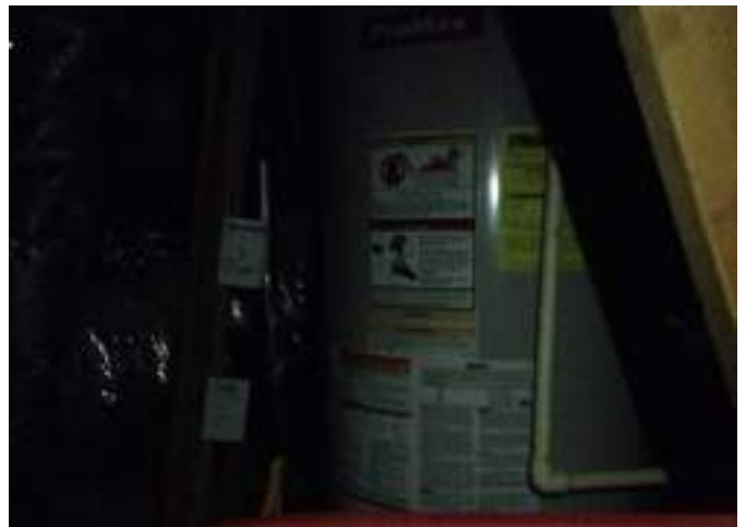
Hot water heater in attic
